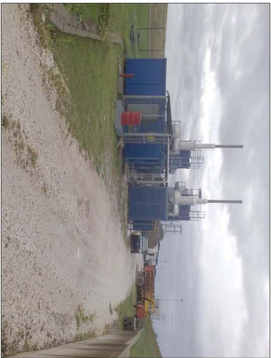
Plant of energy recover from biogas
